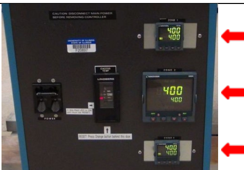
Figure 5: Controls for a 3-zone furnace--three temp controllers
